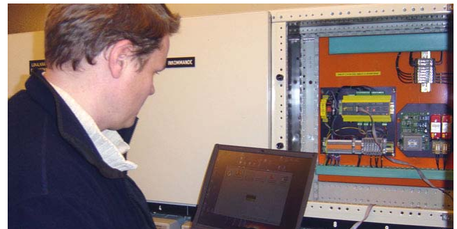
Picture 1 ProTrol IPC4010 integrated controller installation at M1.
